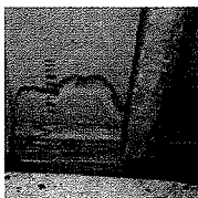
Look for water stains on walls, ceilings, woodwork and other surfaces.
